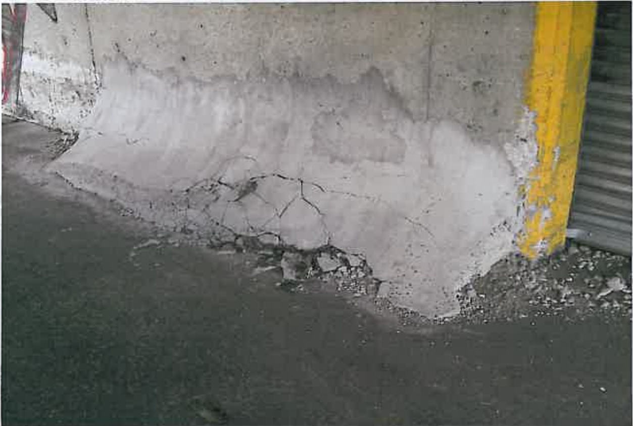
PARTIAL VIEW OF DAMAGED EXTERIOR WALL OF SUBJECT
