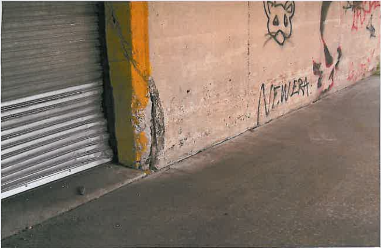
PARTIAL VIEW OF DAMAGED EXTERIOR WALL OF SUBJECT
